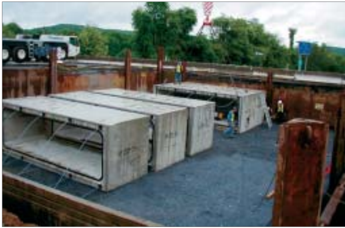
The box culvert, part of the value engineered design change, exceeds the 50-year design and performance standards.
