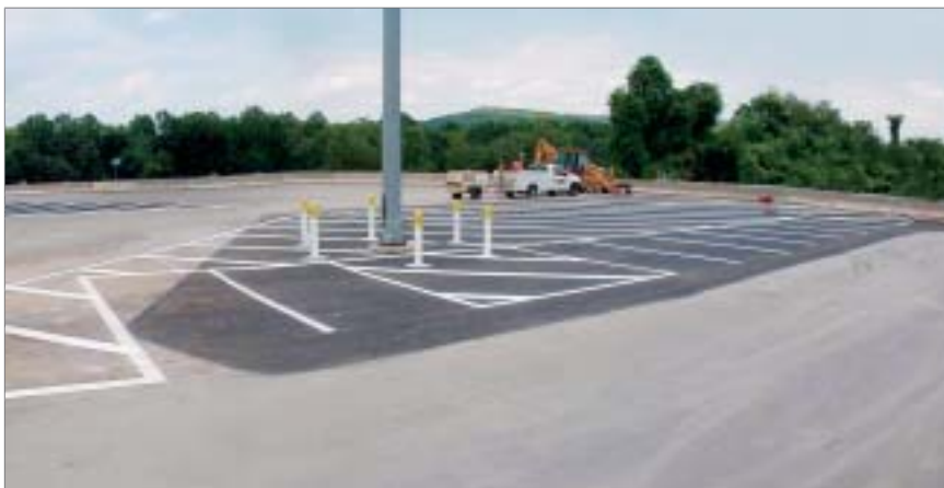
The completed project, on which there are no truck traffic parking prohibitions.
