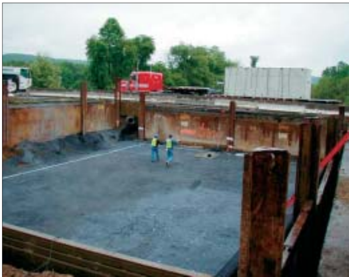
The value engineered design change consolidated all underground detention in one area.
